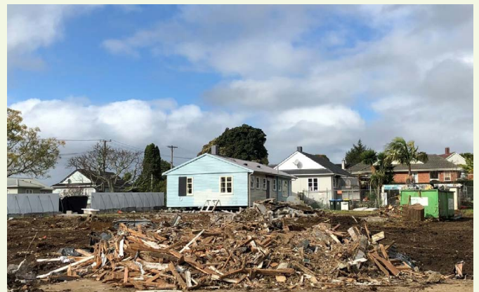
Eight old houses in a Mount Albert development were removed using deconstruction.
