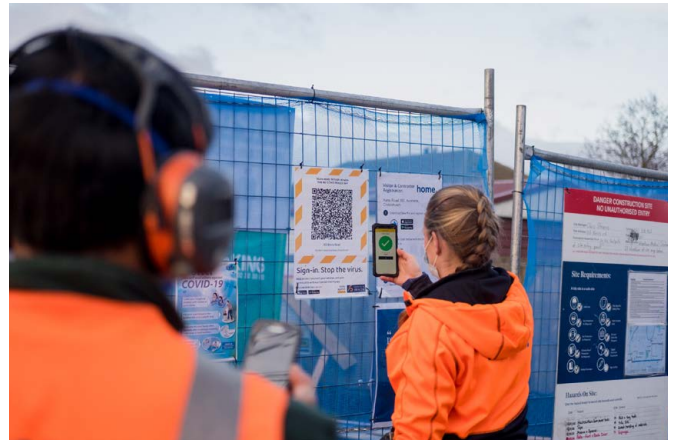
Signing in to enter a Kāinga Ora-Home redevelopment site with the COVID Tracer App.
